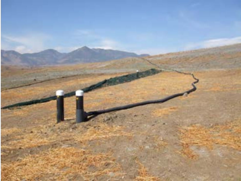
Figure 4. Looking West, at Berm 4 and the Gravity Drain Line Connection to the ESDD
