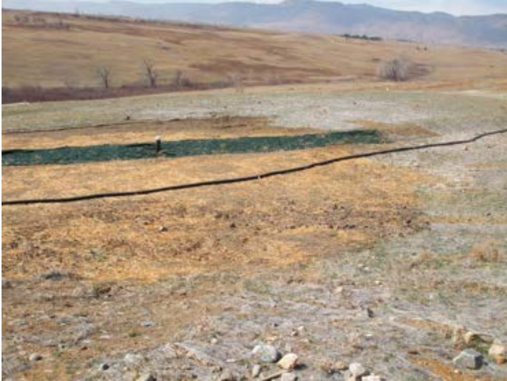
Figure 2. Looking South at Berm 4 and the New Above-Ground Drain Pipe Running from the OLF Groundwater Intercept System to the ESSD
